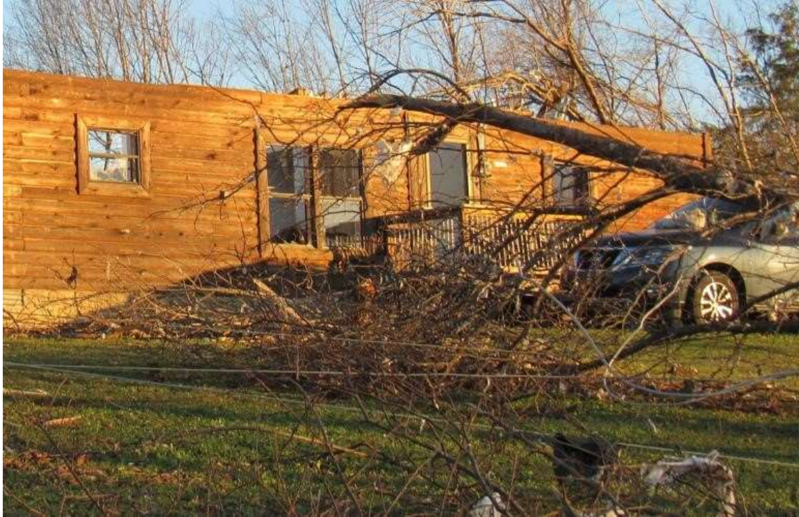
Figure 6 Damage to home and car in SE Cheatham County following the Dec. 11, 2021, tornado outbreak. (Source: Cheatham County Exchange)
