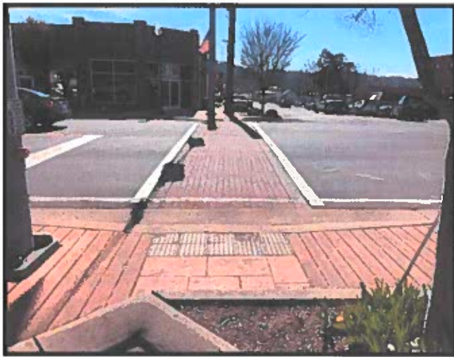
Main St. and Cumberland Pole in Ramp, Deficient Detectable Warning Surface
