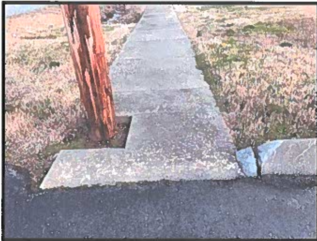
Little Marrowbone Rd. Utility Pole Obstruction
