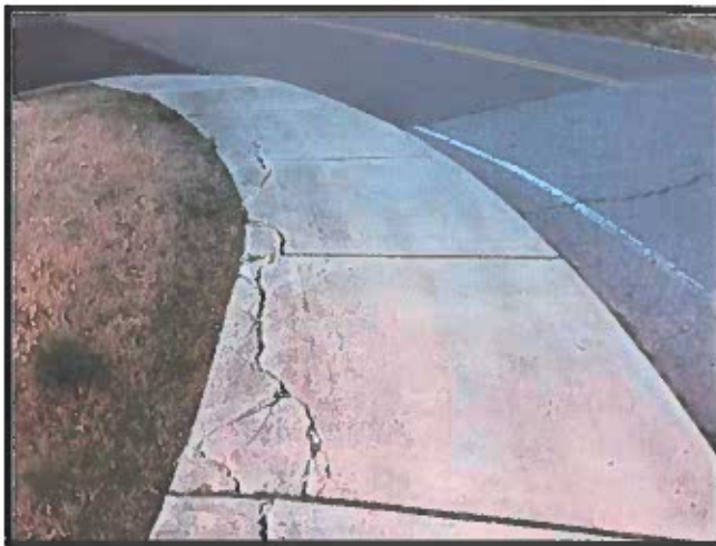
Ruth Street- Cracked Sidewalk and Cross Slope >2%
