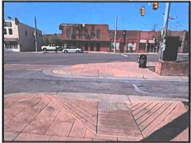
Main St. and HWY 49/Frey St. Excessive Flare Grades, Courthouse Entrance Drive
