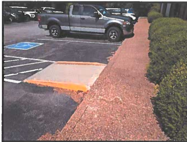
Police, Parks & PW Ramp and Sidewalk Deficiencies
