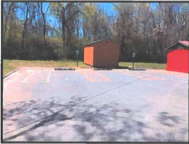
J.W. Johns Jr. Access Aisle & Signage Non-Compliant
