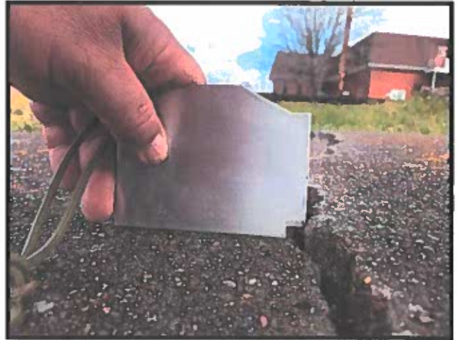
HWY 49/Frey Street- Typical Discontinuity >1/4"
