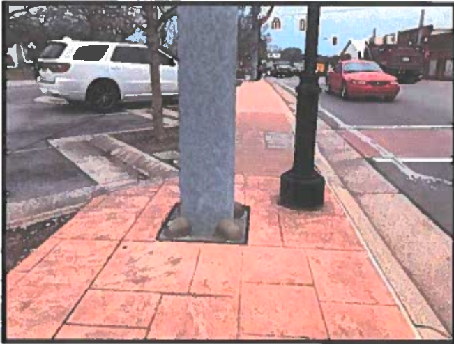
Main Street/HWY 12-Utility Poles Obstructing Path/Ramps
