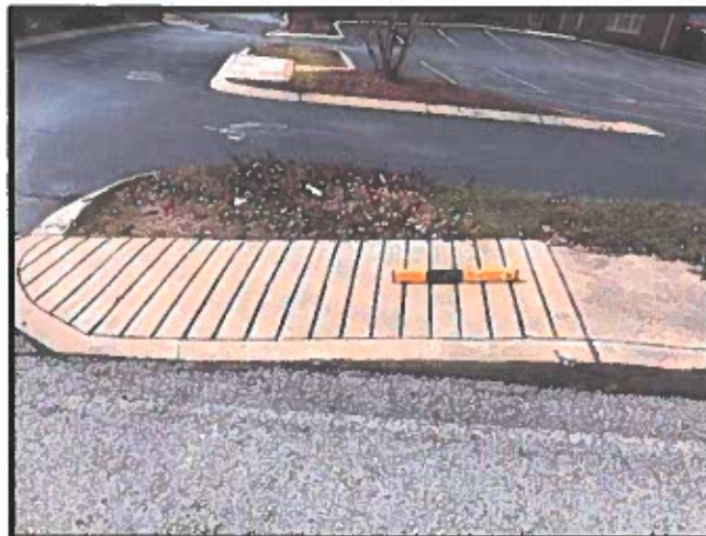
Duke Street- Running Slope of Ramp >8.3%
