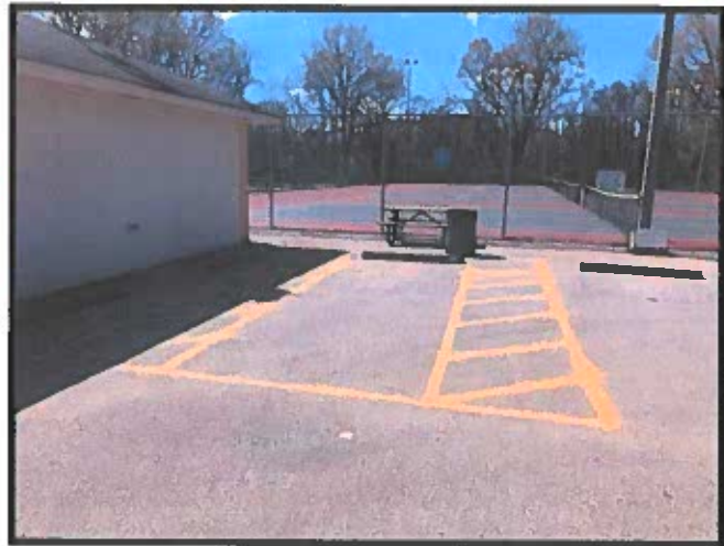
John C. Poole Parking Space & Aisle Non-Compliant
