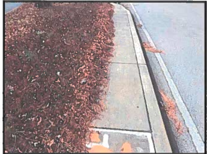
Helen Street- Typical Obstruction Due to Overgrowth
