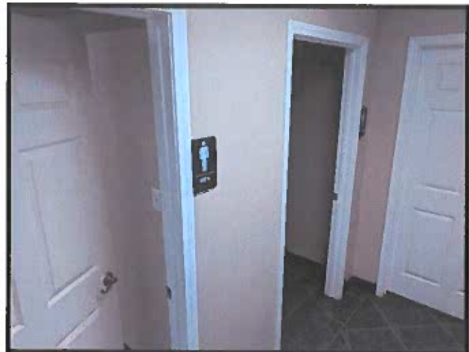
Parks/PW Dept. Restroom, Non-Compliant Signage
