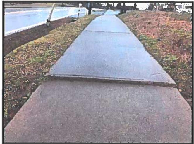
Main Street/HWY 12-Typical Discontinuity >1/4"
