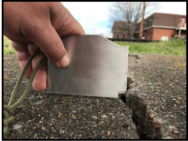
HWY 49/Frey Street- Typical Discontinuity >1/4"
