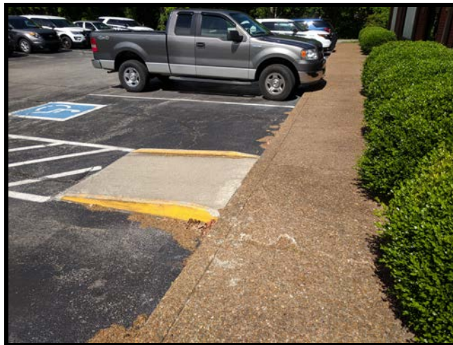
Police, Parks & PW Ramp and Sidewalk Deficiencies
