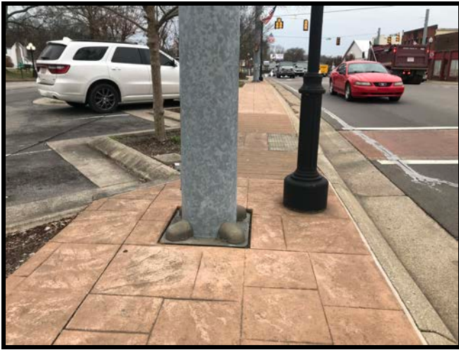
Main Street/HWY 12-Utility Poles Obstructing Path/Ramps
