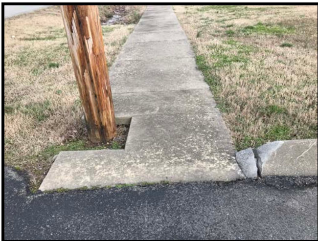
Little Marrowbone Rd. Utility Pole Obstruction
