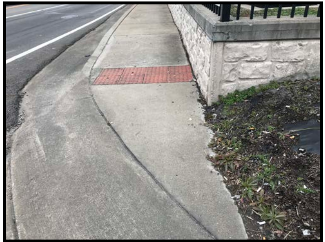
Main Street/HWY 12 No Accessible Ramp, Slope Exceedance/DWS Misplaced
