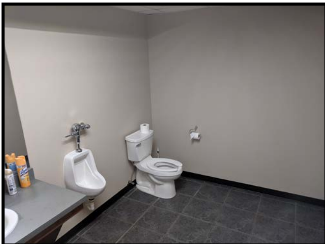
Parks/PW Dept. Restrooms, No Safety Handle
