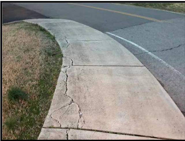
Ruth Street- Cracked Sidewalk and Cross Slope >2%
